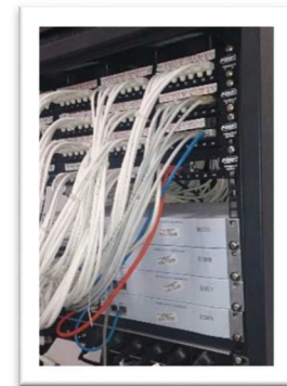
Figura 3-2 - Vista Trasera Patch panel
